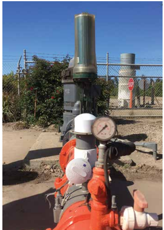
AMI installed on an agricultural well in the Oxnard basin. © Sarah Heard/TNC
