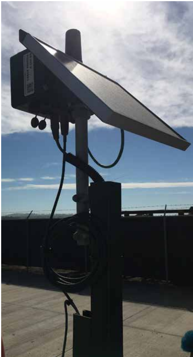
AMI installed on an agricultural well in the Oxnard basin. © Sarah Heard/TNC
